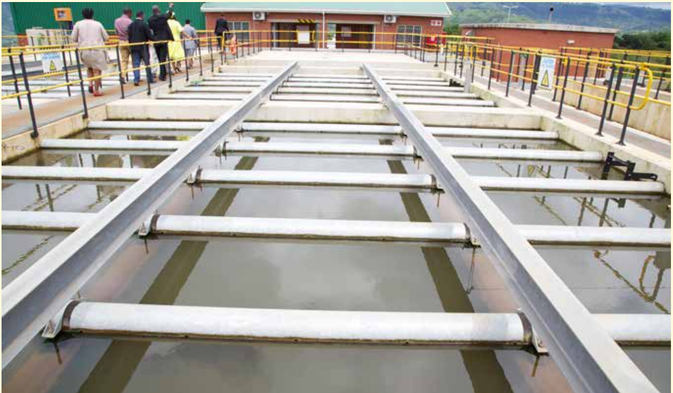
Maphumulo bulk water supply
