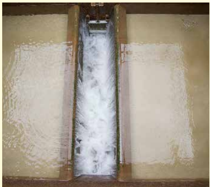
Back wash water purification system in Maphumulo
